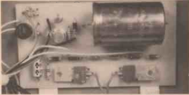
Inside the points switch, note the position of the thyristors
