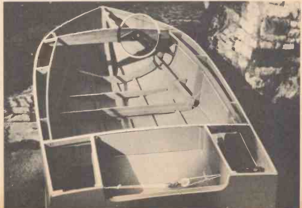
All of the internal structural work has been done. The motor well is complete and remote steering cables have been fitted. The next job is the making of the plywood deck.
