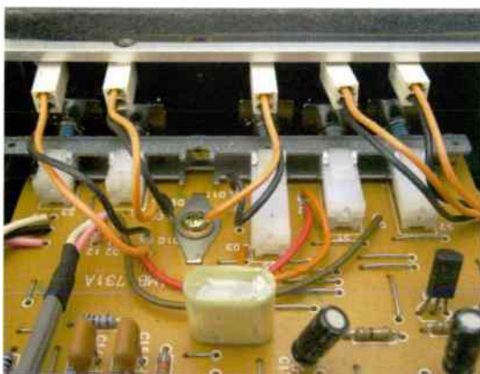
If the switches get a lot of use – to say, compare the unprocessed and processed sound – they wear out. The unit featured here suffered this.
