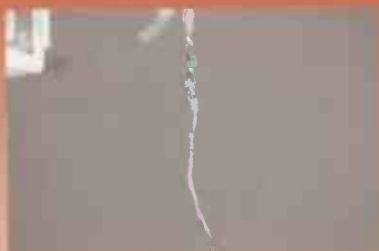
The new wires soldered to the old ones, ready for pulling through.
