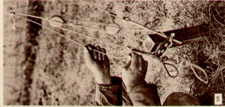
35 Setting up the guy wire with block and tackle on the strainer
