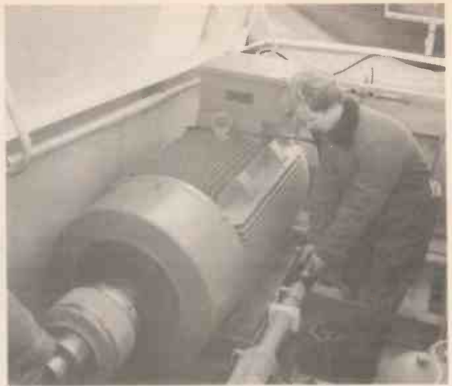
A generator for the V27-225kW turbine.
