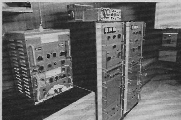
Part of the Redifon installation for Pentagone 84 , showing (l to r) the emergency m.f. radio-telephone, the G543 i.s.b. transmitter and the G452 transmitter for teleprinter work on s.s.b. or i.s.b. The settee beyond these transmitters contains the 24 volt emergency batteries in a sealed gas-tight compartment.
