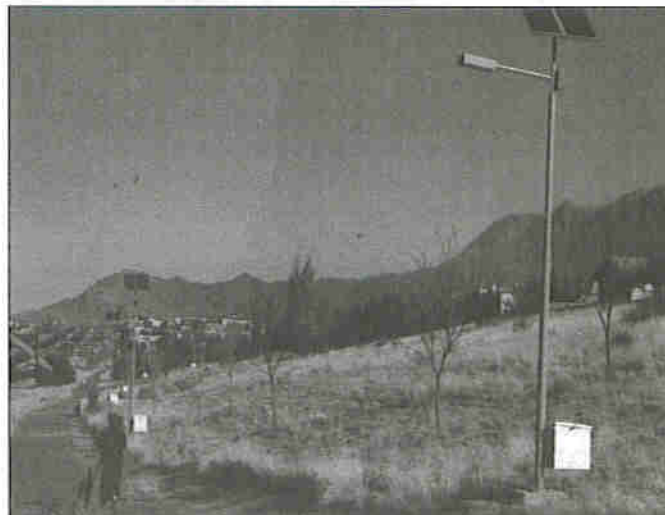
Figure 11: Use of solar photovoltaic systems for street lighting in Albuquerque, New Mexico. (Courtesy US Department of Energy)
