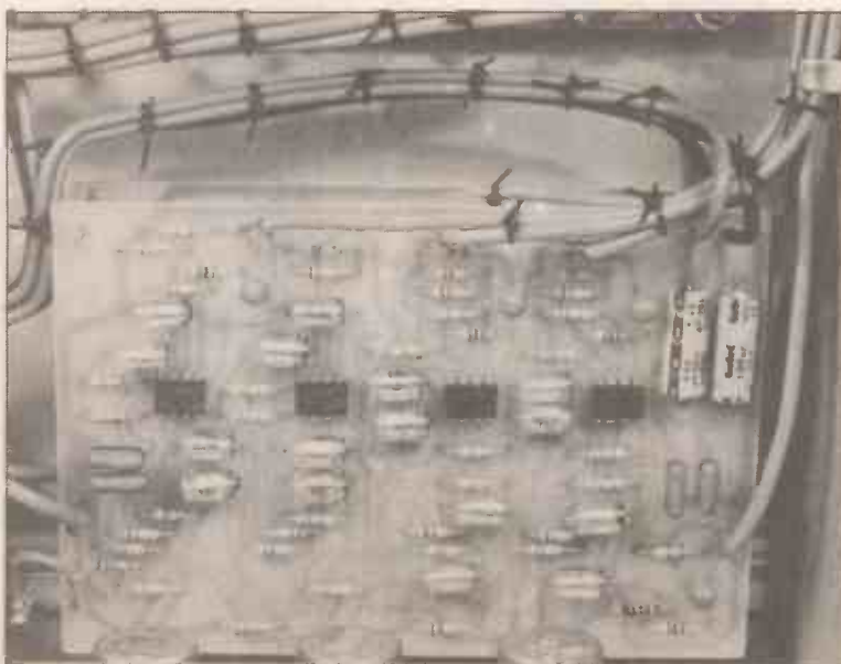
View of Crossover board.
