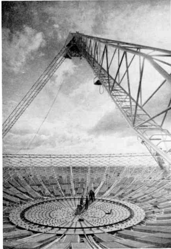
Fig. 3. View of the paraboloid after construction of the spiral purlin system, the centre plating and the erection of the tripod.
