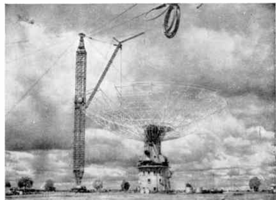
Fig. 2. Final section of the reflector supporting structure being lifted into position (May 1961).
