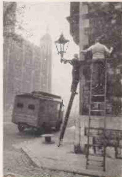
E.M.I. engineers are here installing the new central hidden television aerial installation at the Tower of London which replaces the previous heterogeneous growth of individual aeri-als.
