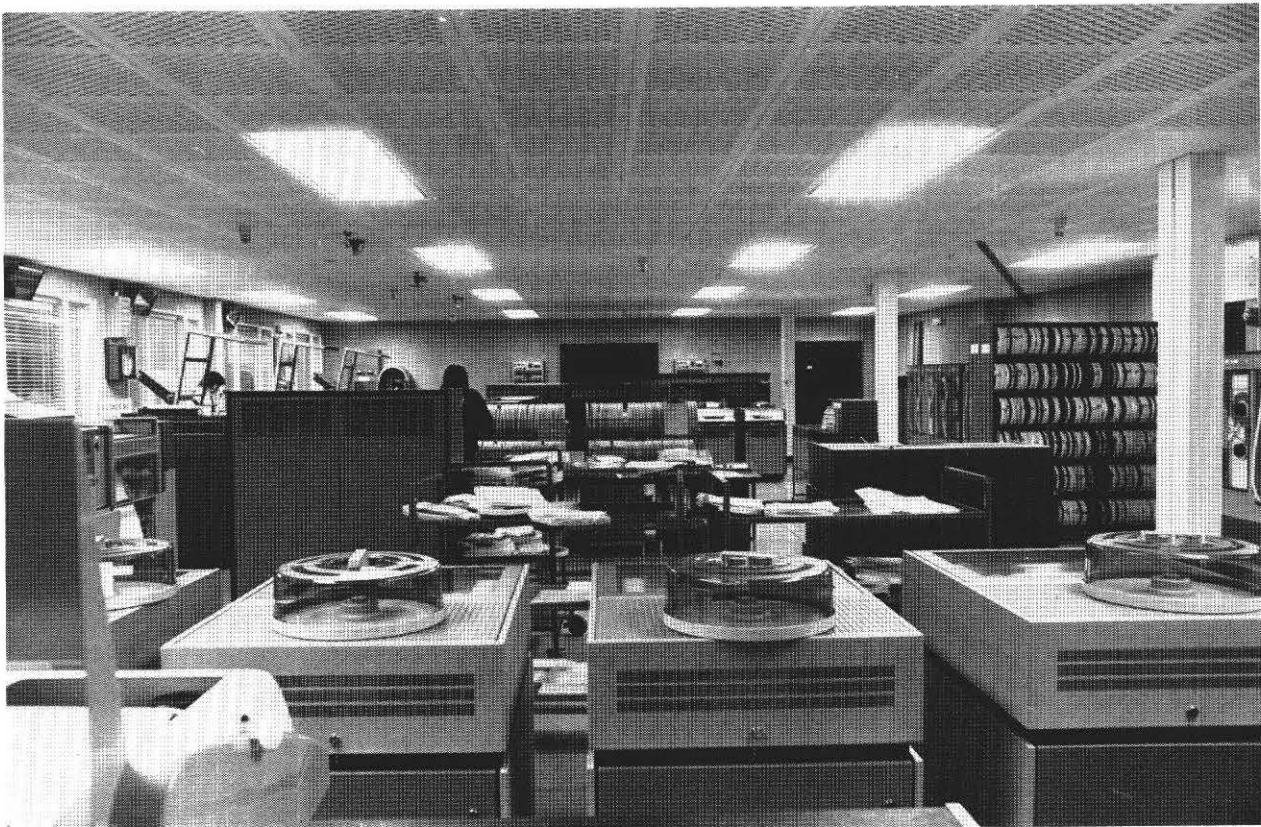
Fig. 1 General view of central computer complex
