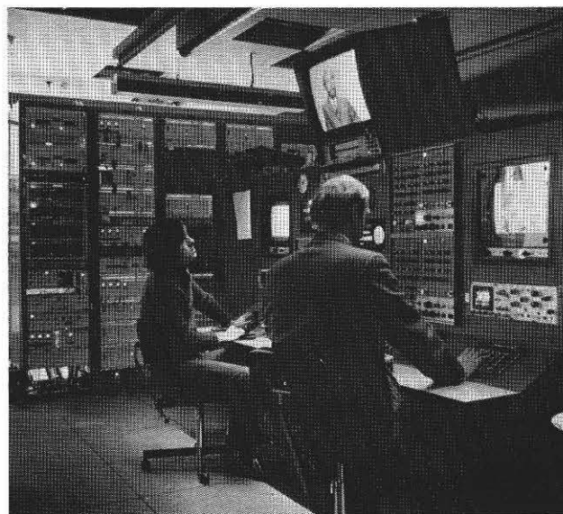
Fig. 3 Television Apparatus Room. In addition to housing the central pulse distribution equipment, this area serves as a common vision apparatus room for both the television studios
