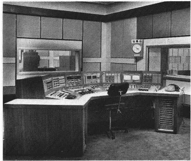
Fig. 6 Radio Studio 1 Control Desk. This is a fully stereophonic 'Type D' installation
