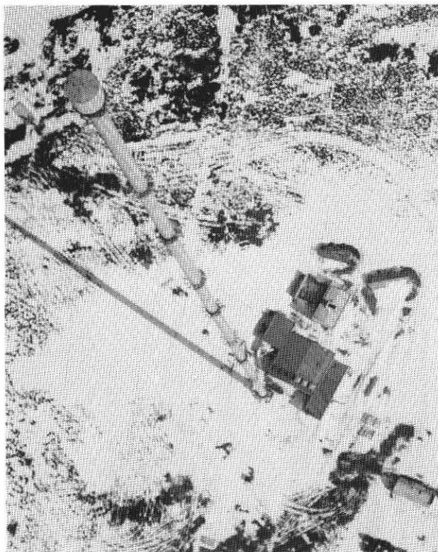
Fig. 10 The mast at Bilsdale West Moor under construction. Even with snow on the ground work continued inside the g.r.p. erection chamber at the top with access via the inside of the mast.
