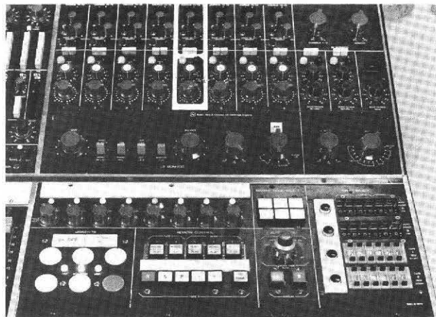
Fig. 4 Part of sound control desk showing, at top, monitoring matrix for MSR, at bottom, remote controls for HVTR and MSR transports, mode and time-code selectors and source switcher.
