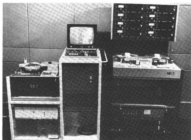
Fig. 3 Helical-scan videotape recorder and multitrack sound recorder used in 'Dub to Sypher'. Similar equipment is used in the control room for 'Sypher dub'.
