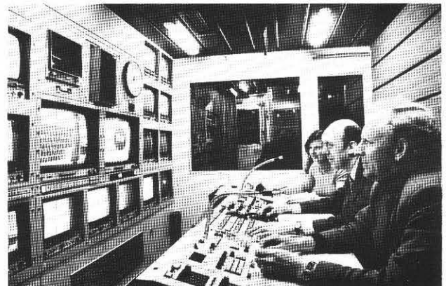
Fig. 5 Type 4 CMCR: Production Control Room
