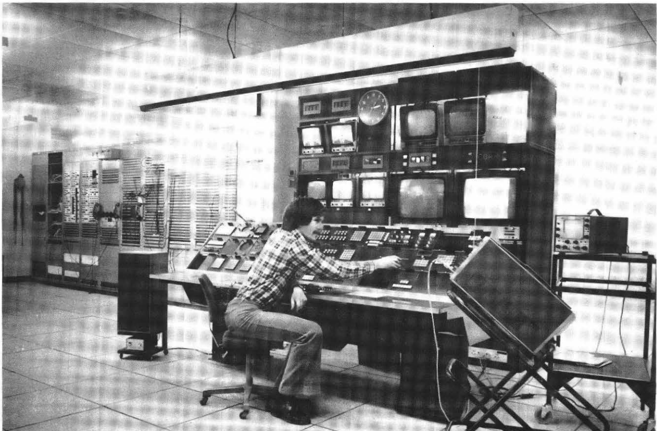
Fig. 10 The control desk in the Central Technical Area
