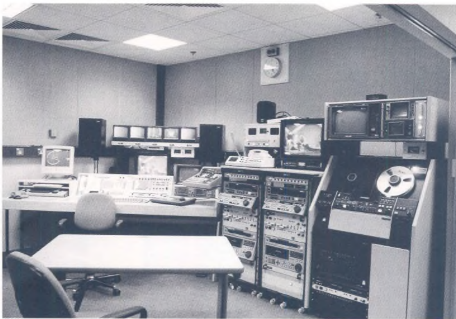
One of the general-purpose VT cubicles (2nd floor).
