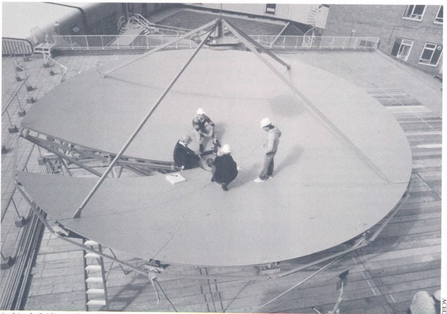
Applying the finishing touches to the dish before the final hoist into position.
