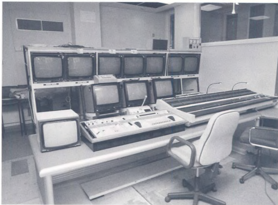
Lighting Control Room showing Galaxy and Celco desks running in parallel.
