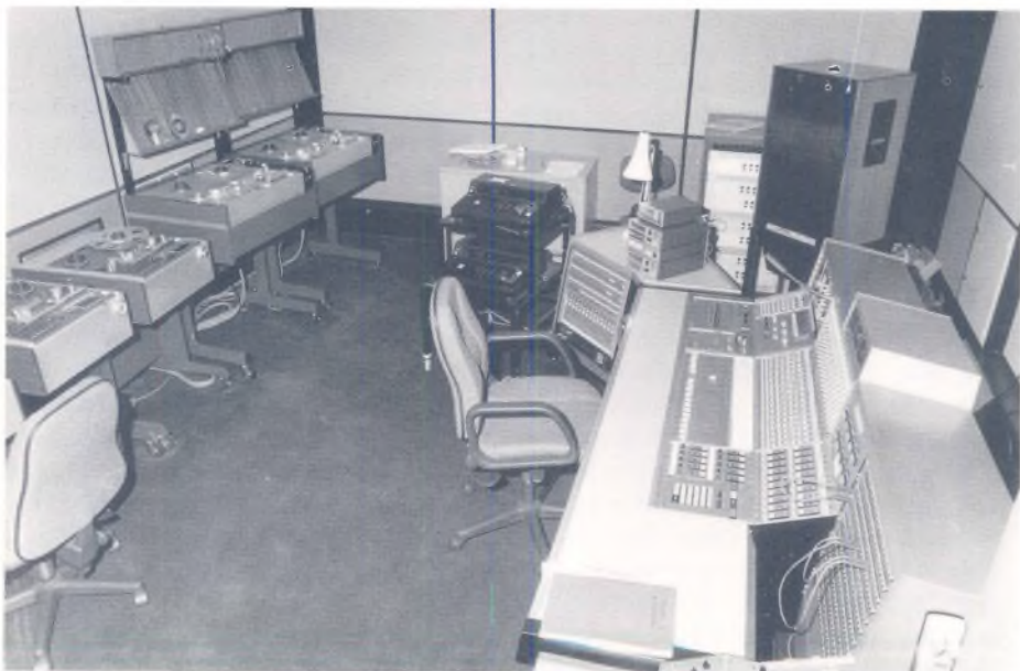
The refurbished control room of Pebble Mill 5
