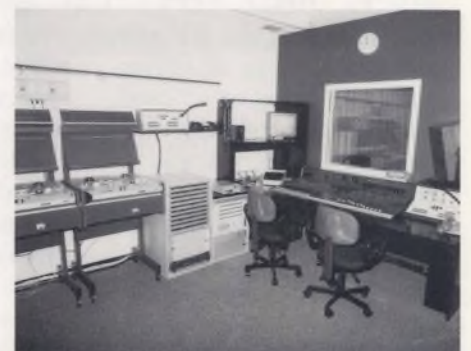
Control room of one of the CBA radio studios.
