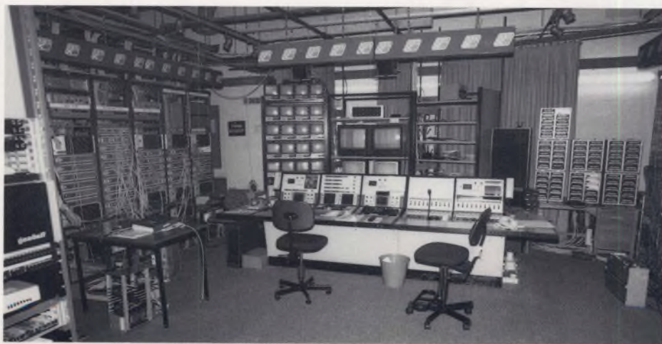
CTA control desk during the working-up period.
