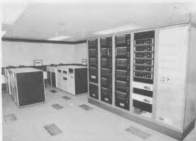
General view of MSS computer room
