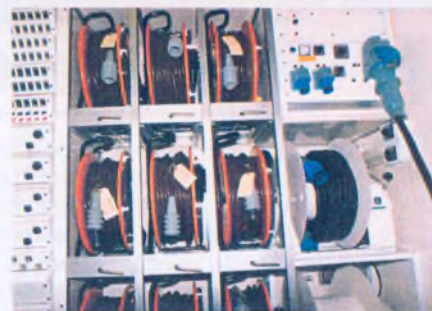
Rear cable storage
