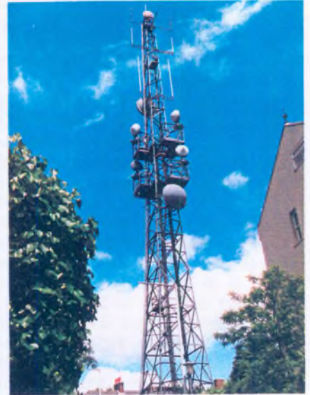
Swains Lane, showing five rotating SHF aerials - 1 at the top and 4 half-way down
