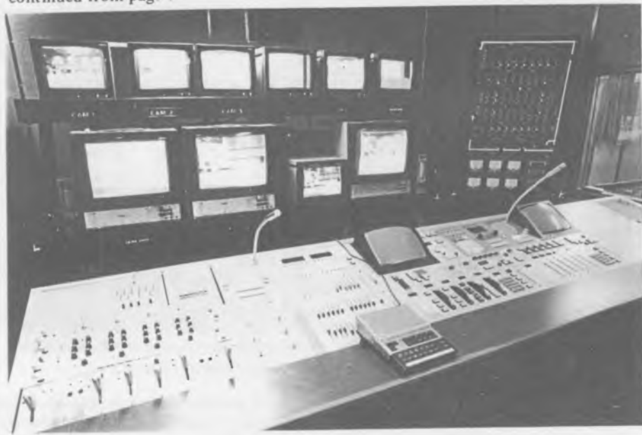
TV Studio 1 Vision and Lighting Control Room with Vision Control Panel (left) and Thornlite 500 with its mimic display.
