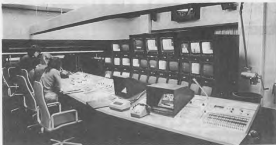
TC2 Production Control Room
