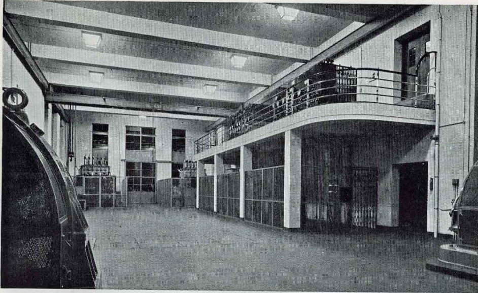
THE HIGH-TENSION MACHINE ROOM, TAKEN AT NIGHT, SHOWING THE A.C. INPUT SWITCH-BOARD, SMOOTHING ENCLOSURE, AND THE TWO MERCURY-ARC-RECTIFIER ENCLOSURES
