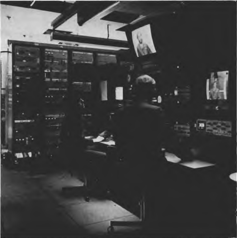
Television apparatus room, Birmingham Broadcasting Centre, 1971
