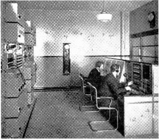
THE AMPLIFIER BAYS AND CONTROL POSITIONS IN THE NEW CONTROL ROOM AT LEEDS
