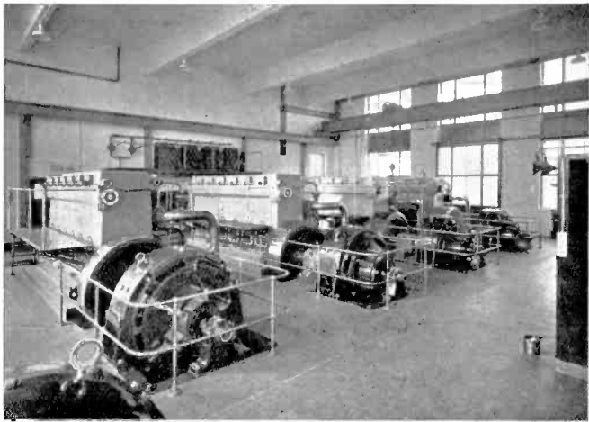
THE POWER HOUSE SHOWING THE FOUR DIESEL ENGINES AND GENERATORS
