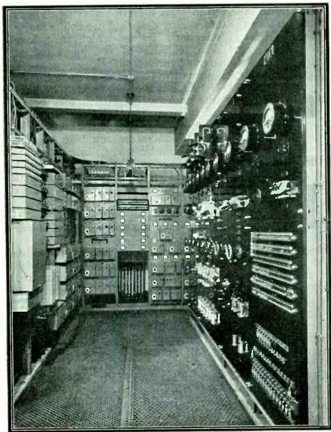
ANOTHER PART OF THE CONTROL ROOM AT MANCHESTER
