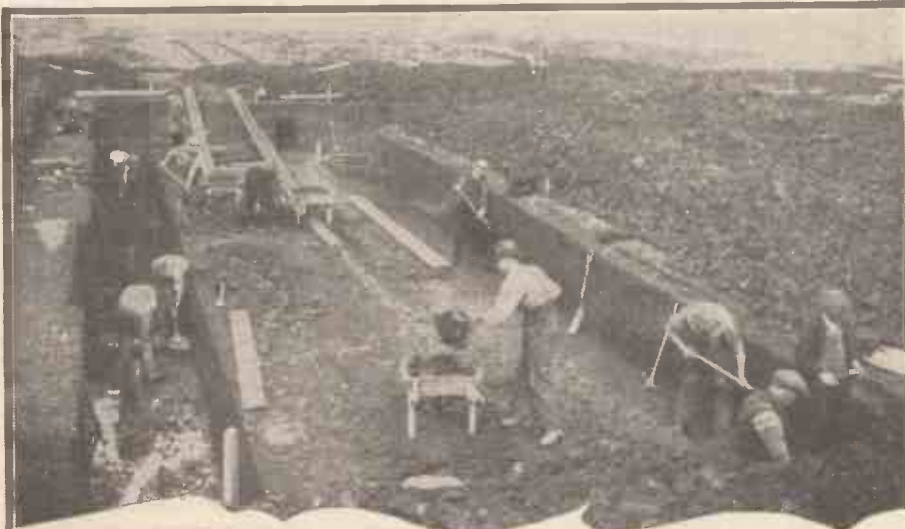
Rapid progress is being made at Washford Cross, where work is in hand for the new West Regional transmitter. The excavations are here being made for the foundations to carry the building and the heavy machinery
