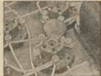
Small components such as coupling condensers can sometimes be connected directly between valve holders
