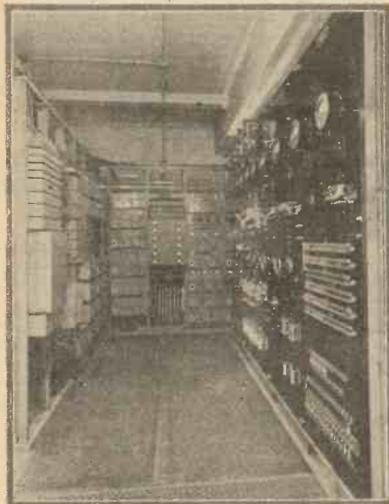
The back of a control room panel. The amplifiers are in the shielded boxes on the left and at the end of the passage, and the batteries are controlled by the switchboard on the right. This is the gear installed for test at Manchester before fitting the new control panels in Broadcasting House.
