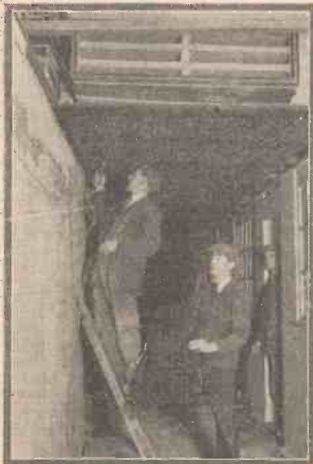
Putting the finishing touches to the sound-insulating and ventilating layers in the corridors of Broadcasting House
