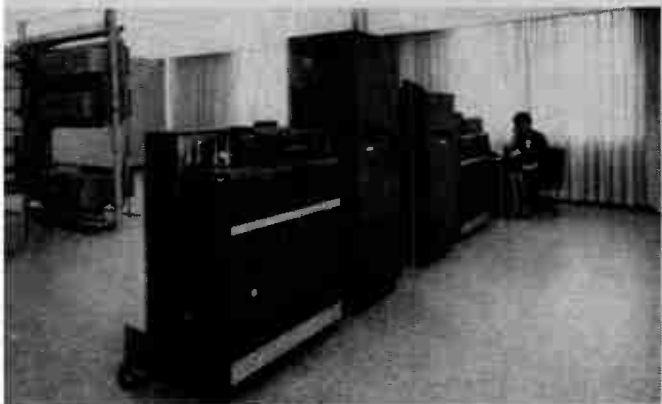
Figure 1. The Collins "Kineplex" communications center . . . equipment is used to transmit mass of business data to remote computer at head office which returns processed information for daily operation of the plant.
