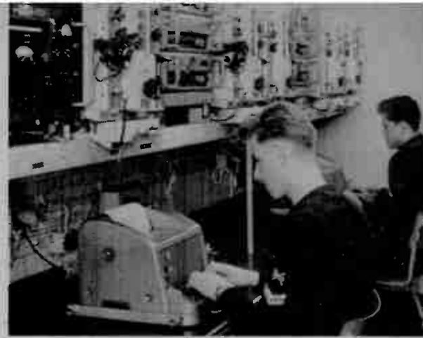
Creed Model 75 teleprinters aboard an aircraft carrier of the Royal Netherlands Navy operate over radio circuits when at sea and can be connected to dockside landlines when ship is in port simply by throwing a switch. This equipment is also in service or on order in over 40 countries.
