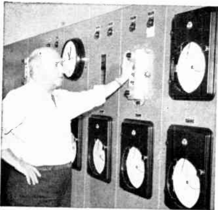
Bell Telemetering channels transmit information to and from this control centre shown above, operating the regulators and valves that handle the flow of gas into and through most parts of metropolitan Toronto.
