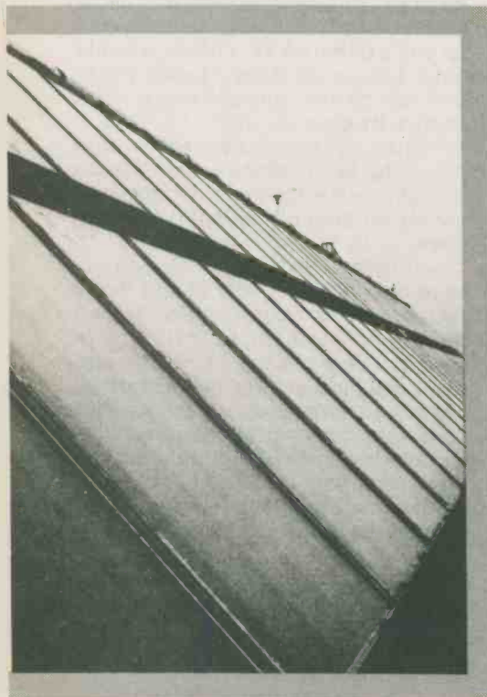
South facing solar panels.
