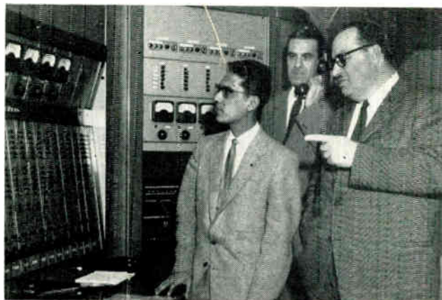
Harry (left) inspecting the automatic network switching facilities in Master Control, Radio-Canada Building, Montreal, with Senior Operator Tam Derbyshire and Assistant Operations Manager Gerry Hudon.
