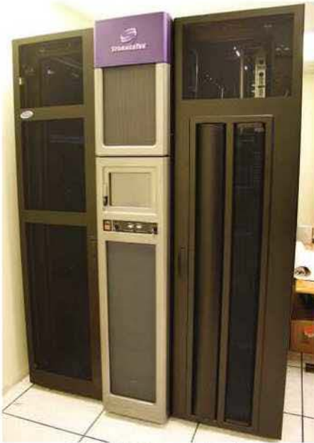
The SUN Storagetek units
