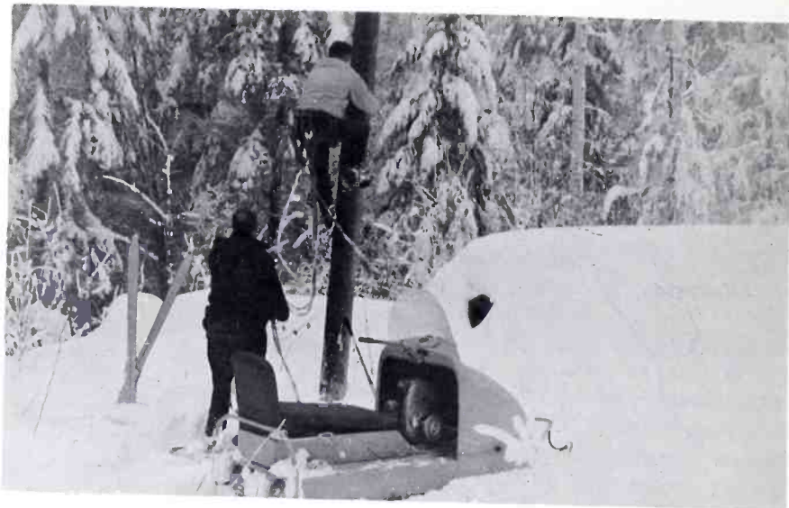
CHBC-TV's intrepid engineers make powerline repairs at 4000 feet, after rampaging up a mountain side on a "skidoo" — a ski-mounted, track-driven vehicle that's become an essential mode of travel in the deep winter snows of the Okanagan ("Paradise") Valley.
