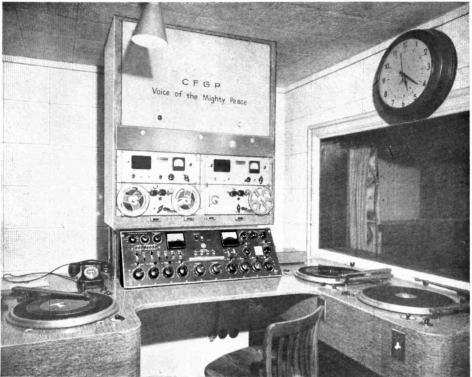
RCA Type BC6A dual channel broadcast console as installed in station CFGP Grande Prairie, Alta.
