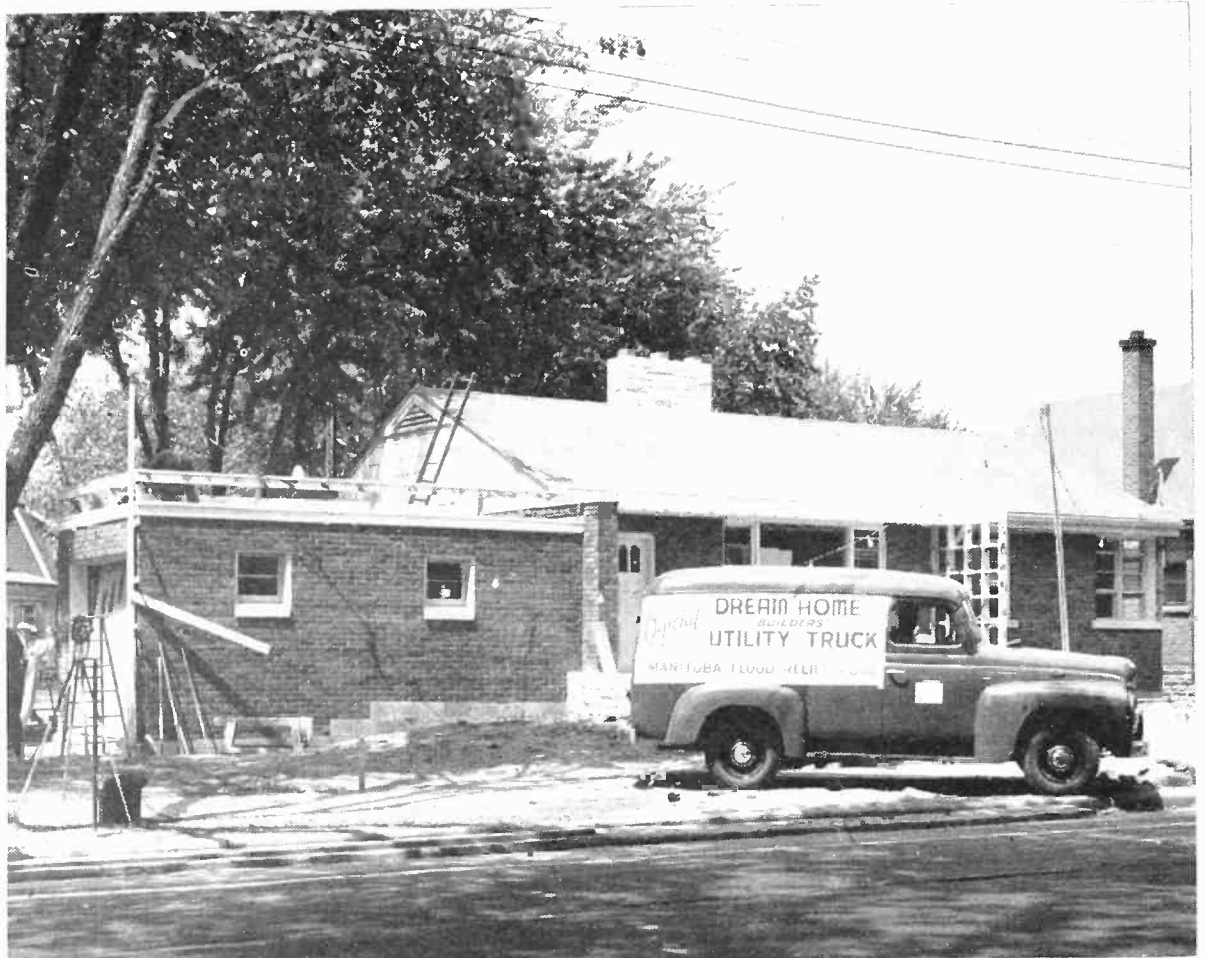
ONE OF THE MOST SUCCESSFUL public service projects in the history of radio was the "Dream Home" built in Hamilton at the instance of CHML president Ken Soble and raffled for nearly a quarter of a million dollars at a dollar a ticket in aid of the Manitoba Flood Relief Fund. Started as a CHML project it gathered such momentum that Soble turned it over to the city. Winnipeg Mayor Coulter flew to Hamilton to present the keys to the house and a new Studebaker to the winner. Everyone pitched in to build the house, from suppliers to men on the job, and the house was erected and lavishly furnished without cost whatsoever in about eight days.
