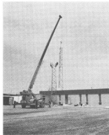
Schindler Communications installs the STL and communication tower at the new CKTY/CFGX-FM complex.
