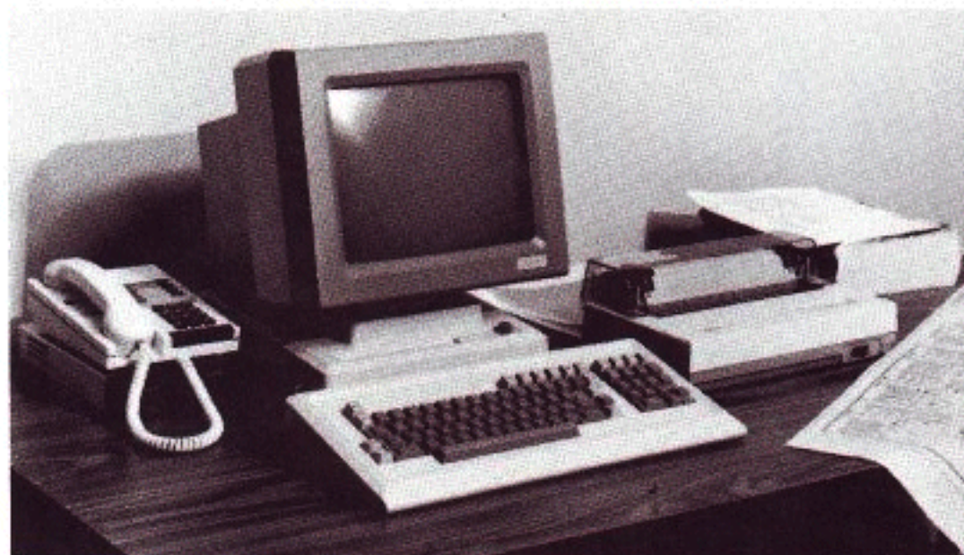
Computerized remote control unit constantly monitors status of transmitting equipment at the CN Tower in Toronto. Terminals use regular telephone lines and are located at studios in both Toronto and St. Catharines.
