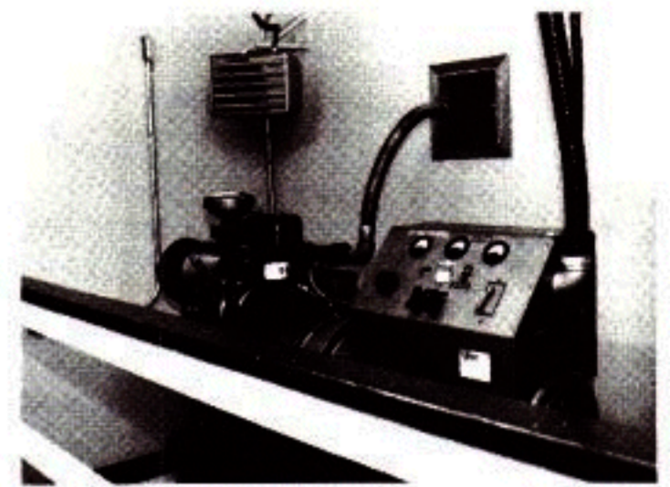
Generator. 25 kw diesel generator is capable of operating the essential services in the building (we did not include management and sales; let them 'freeze in the dark'— or go out and sell!) This plant is essential, since much of our coverage extends to isolated communities where CHCM is regarded as an essential link during extended Power outages.
