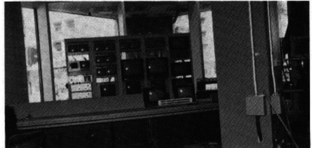
installation crew was busy installing the video control room, which along with activity inside and outside the building is part of the on-air synergy of the Citytv/MuchMusic style. Outside, 'Speaker's Corner' videotapes views of passers-by on topic of day.
