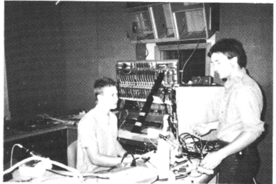
Technicians Geoff Dane and Walt Juchniewicz are seen wiring one of the two full production studios. The studio design for CHML/CKDS-FM is by architect Lionel Mincoff of Montreal, who is a specialist in acoustics.
