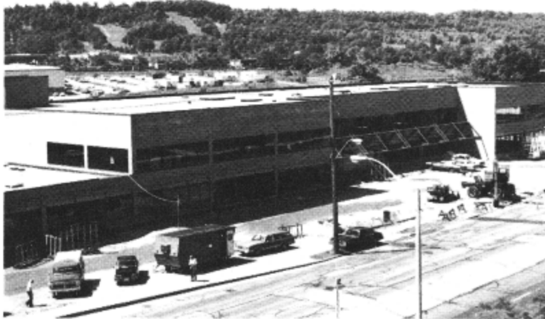
Commercial complex which houses CHML/CKDS is seen under construction at 875 Main Street West in Hamilton. It is opposite Westdale Secondary School and replaced another local landmark, Paddy Greene's pub.
