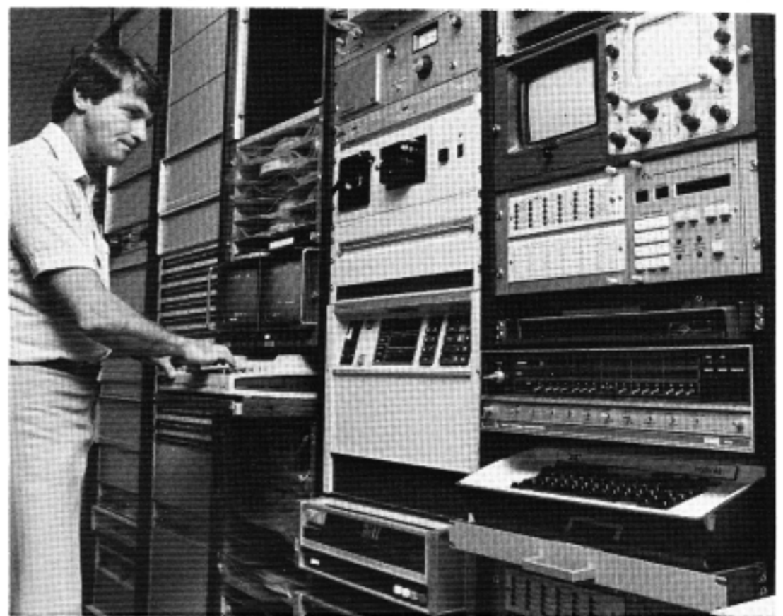
Part of Central Equipment Room
