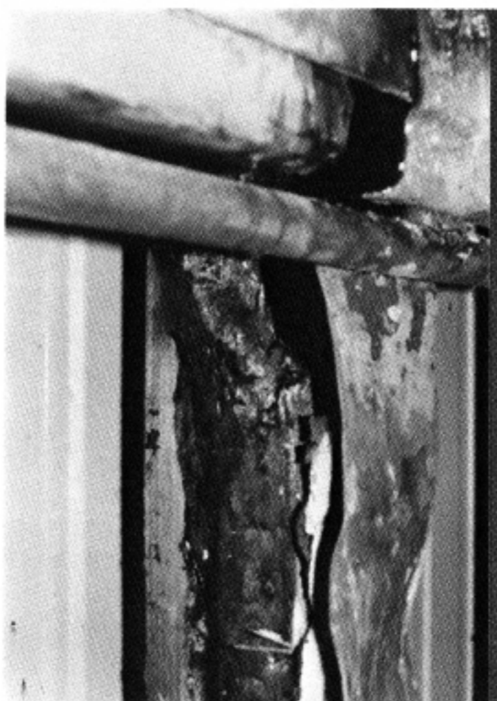
Close-up of conduit and ground strap, CFRB ATU hut. Photos by Bruce Dingwall.
