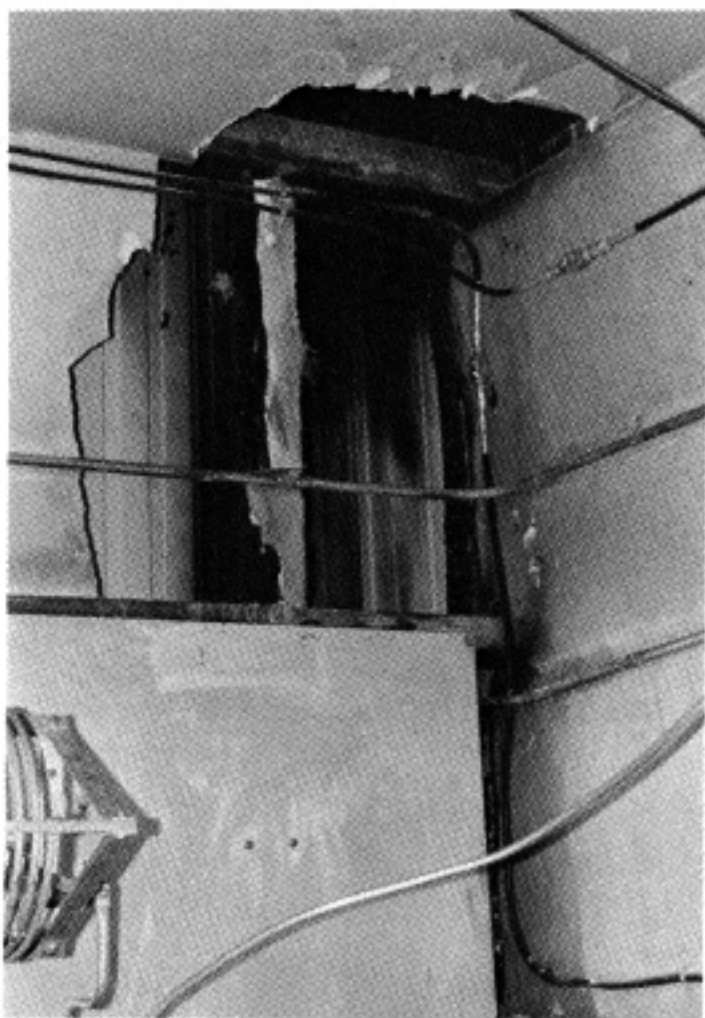
CFRB ATU hut #5, where fire travelled up wall from conduit and ground strap.
