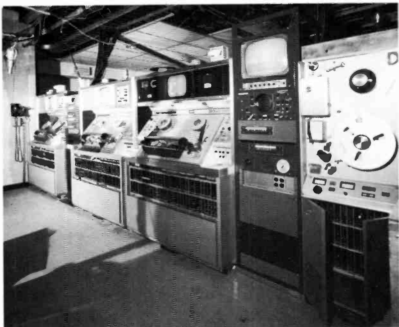
Fig. 8-21. VTR room at WTAE-TV.
