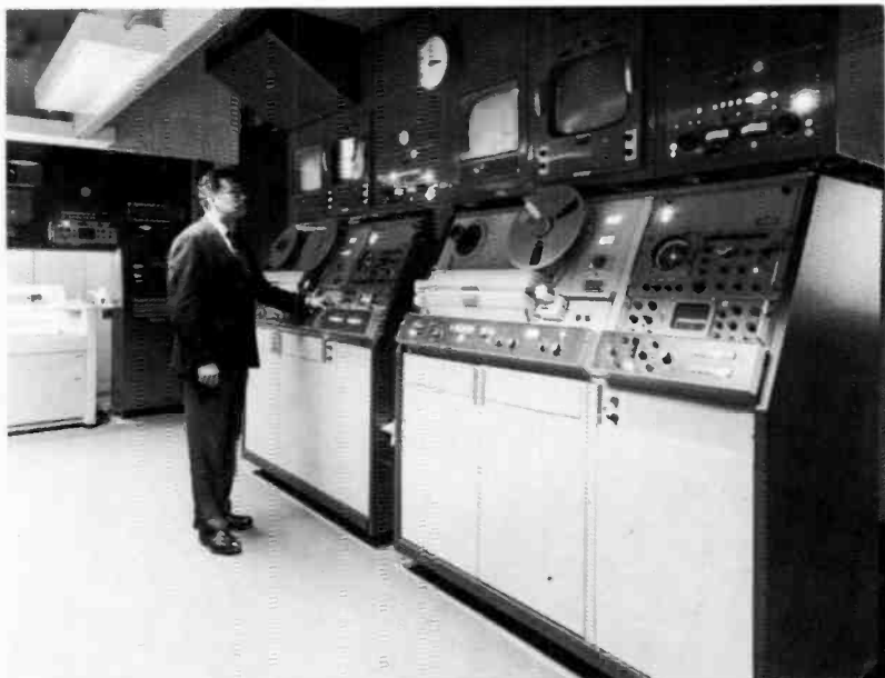
Fig. 8-22. VTR room at WBBM-TV.
