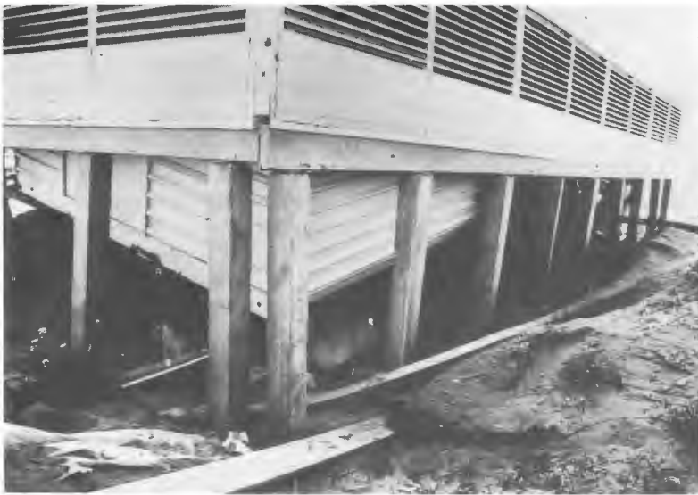
Figure 43.23 Equipment building collapse following erosion of foundations
