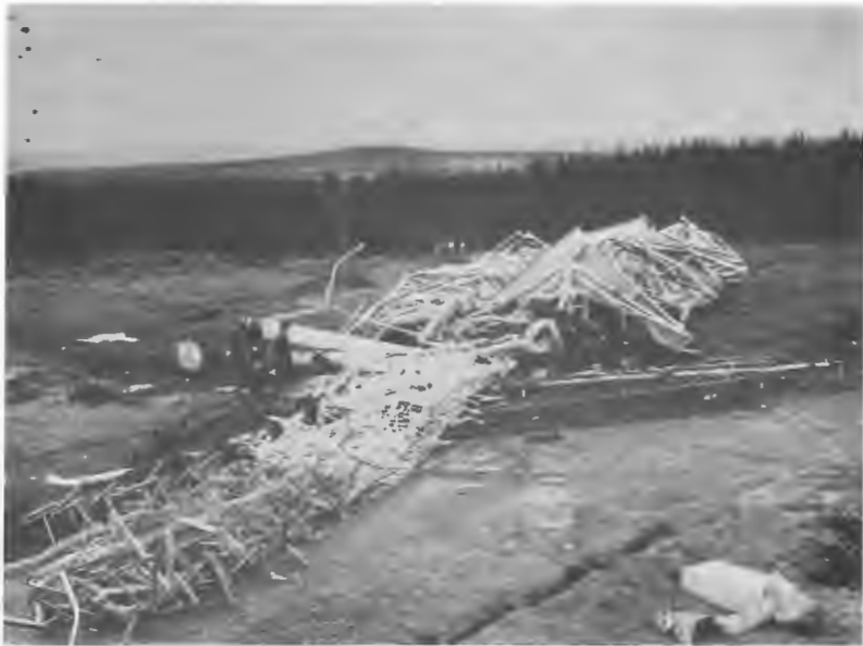
Figure 30.11 Damaged antenna panels and steelwork
