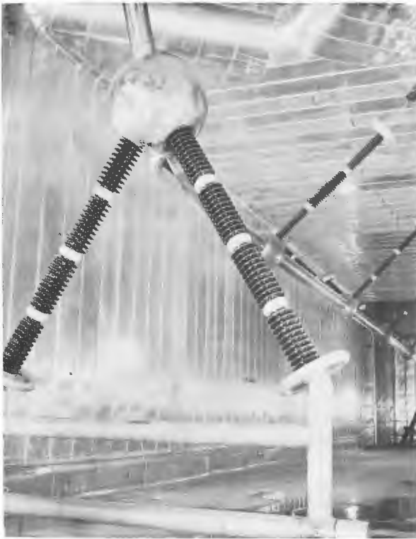
Figure 27.4 Room shielding at 2 MW VLF station (Courtesy US Navy)
