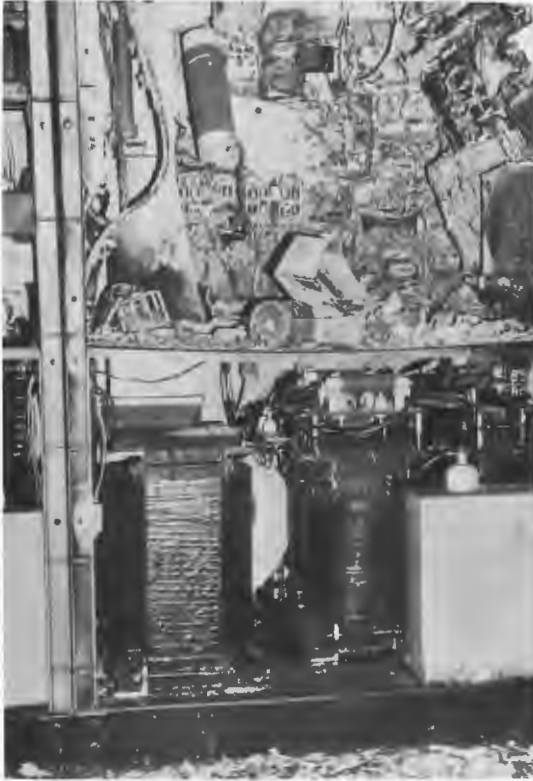
Figure 39.6 Extent of damage in the upper and lower compartments
