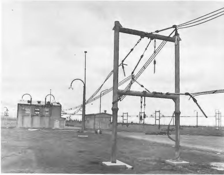
Figure 43.15 Damaged transmission line
