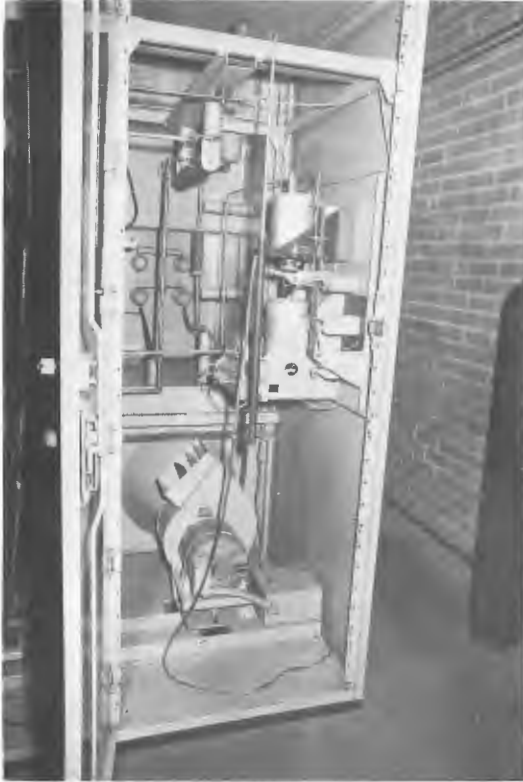
Figure 41.13 Enclosed vault equipment cubicle with transformer entry at rear and forced air cooling
