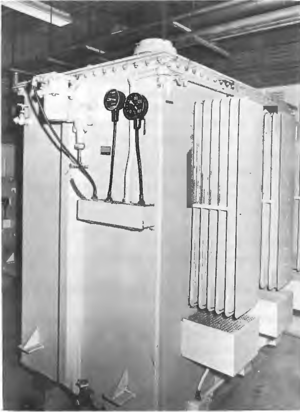
Figure 29.2 E.H.T. transformer of high power transmitter
