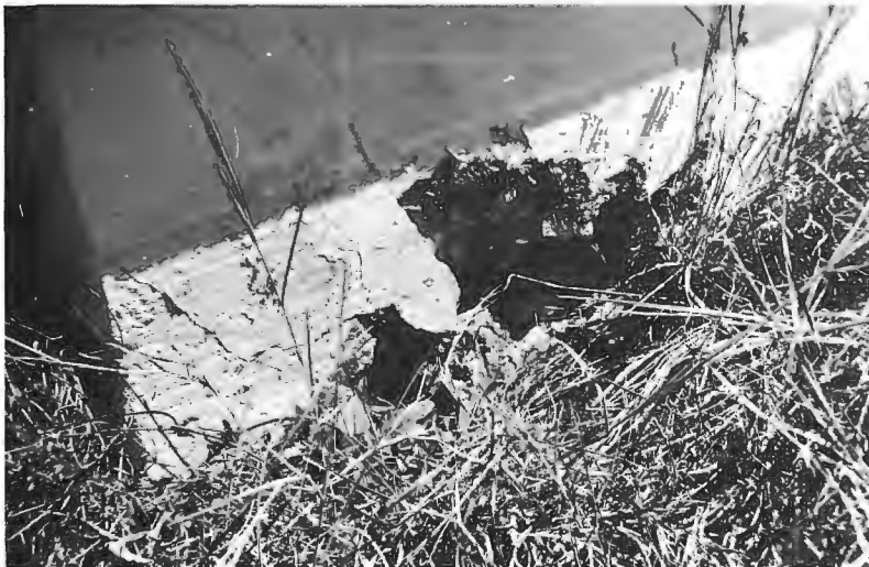
Figure 39.13 Damaged tower footing
