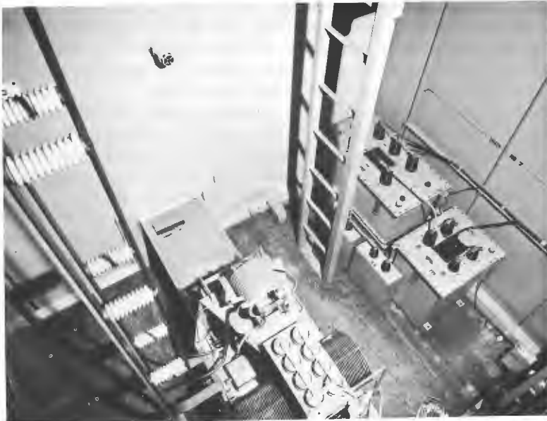
Figure 34.1 Smoke detector inside transmitter cubicle
