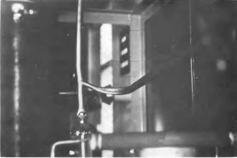
Figure 38.13 Crushed copper tubing of matching equipment
