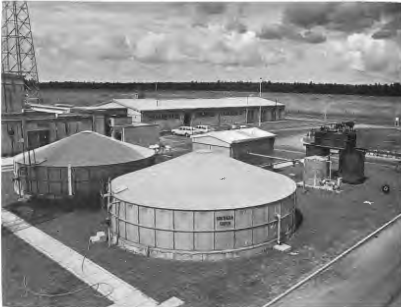
Figure 34.7 Water tank storage and fire pump house
