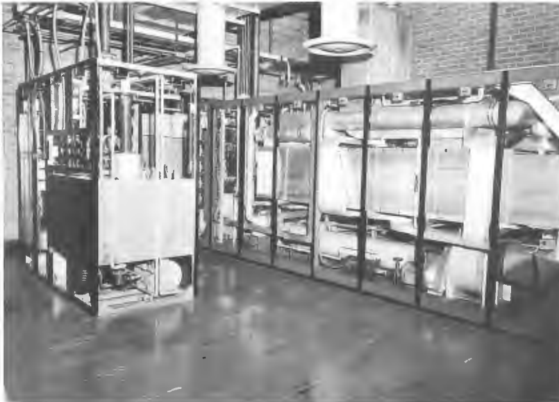
Figure 48.3 250 kW transmitter prepared for visual inspection during acceptance testing
