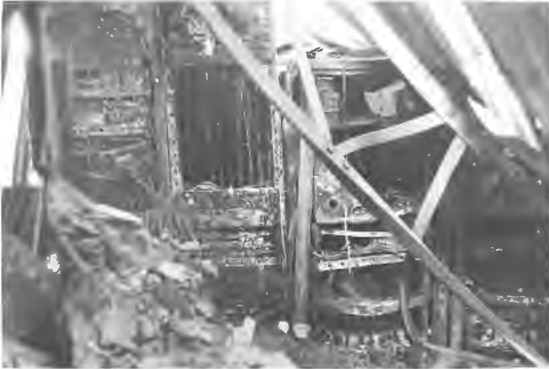
Figure 39.8 Front of transmitter cabinets and racks
