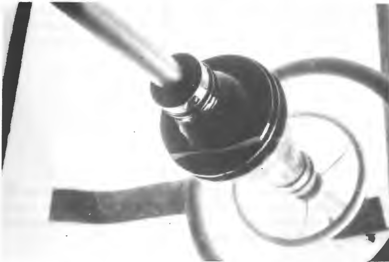
Figure 39.12 Broken skirt on lead-through insulator
