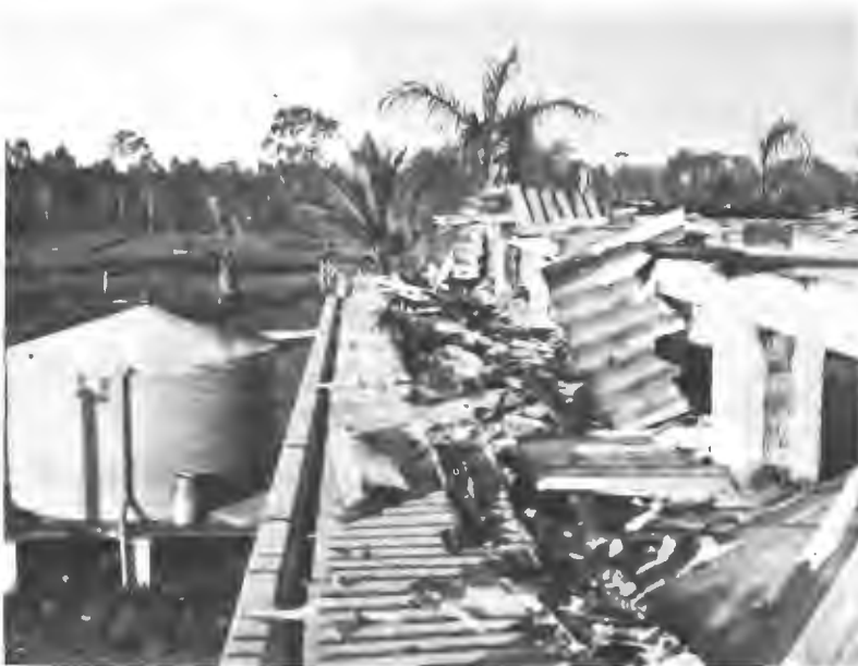
Figure 39.3 Fire damaged transmitter building
