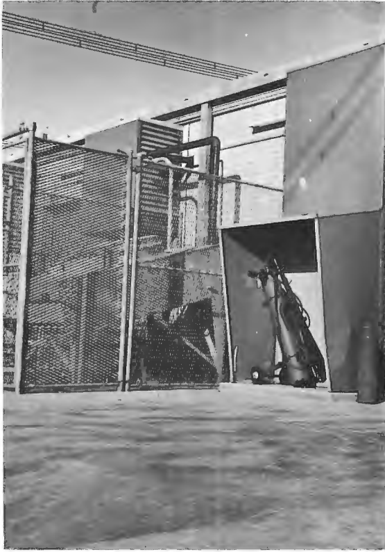
Figure 34.4 Mobile CO 2 units for transmitter and vault areas
