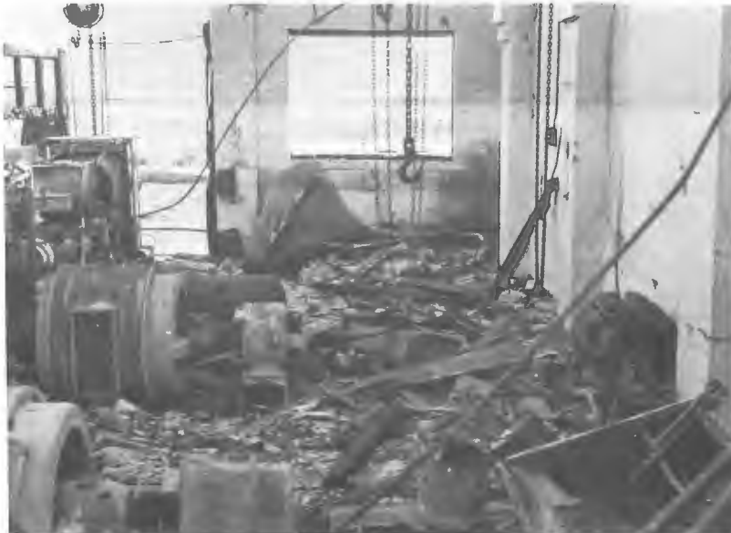
Figure 33.5 Damage in power generating room
