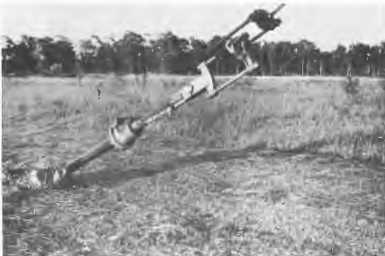
Figure 26.12 Broken guy insulator
