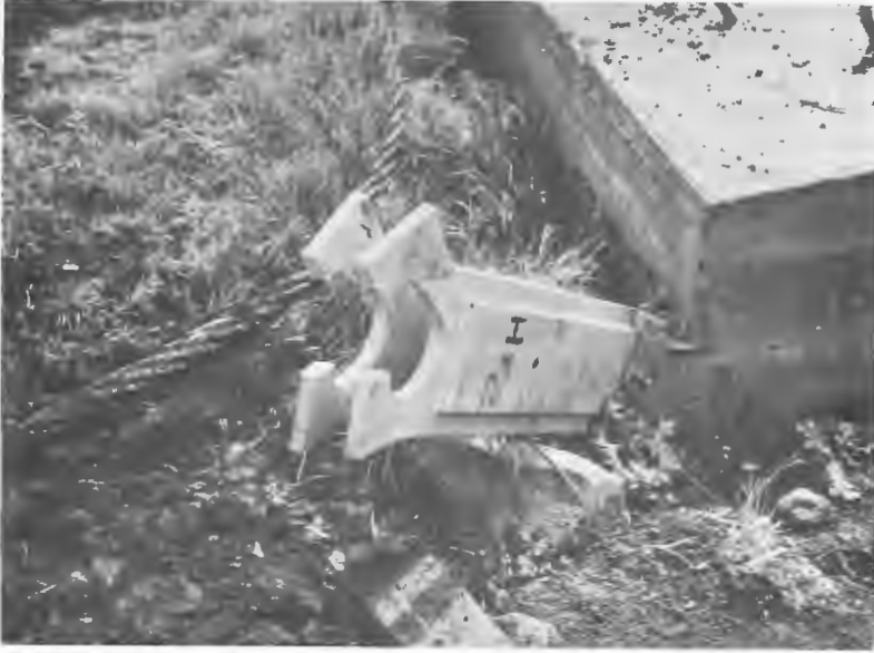
Figure 30.10 Fractured guy anchor strap
