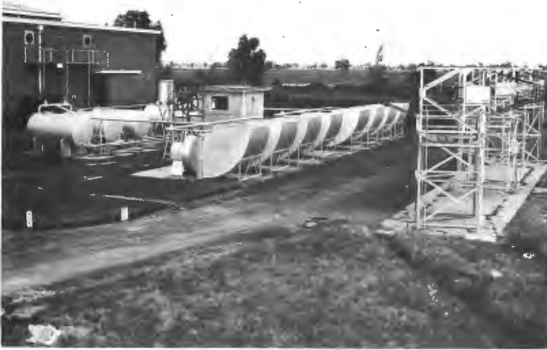
Figure 42.1 Heat exchangers and storage tanks of large water cooling system
