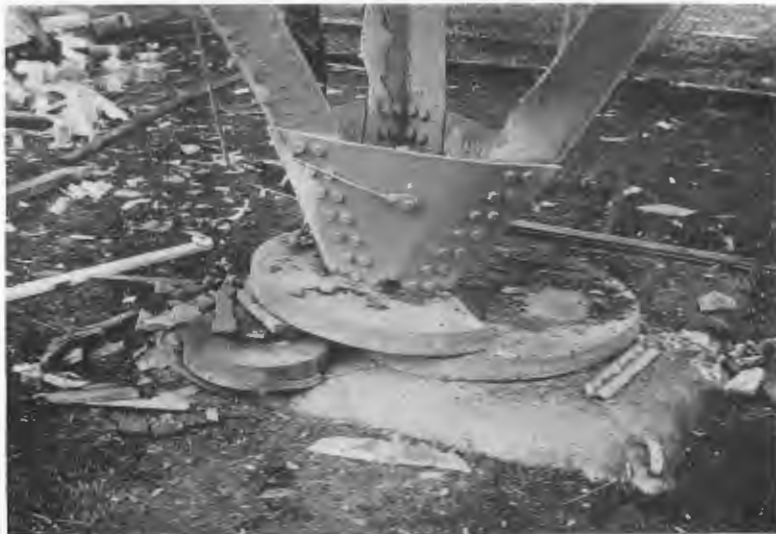
Figure 26.10 Damage at mast base
