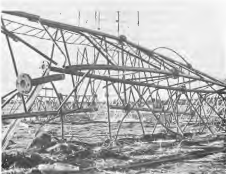
Figure 30.13 Broken solid members and tower in background (Courtesy KHQ)
