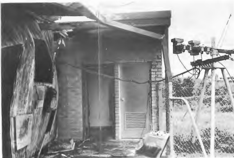
Figure 39.7 Damaged transmitter building
