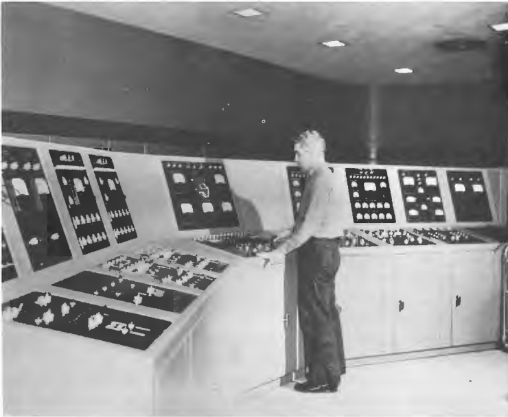
Figure 21.1 Control console of 2 MW transmitter (Courtesy US Navy)
