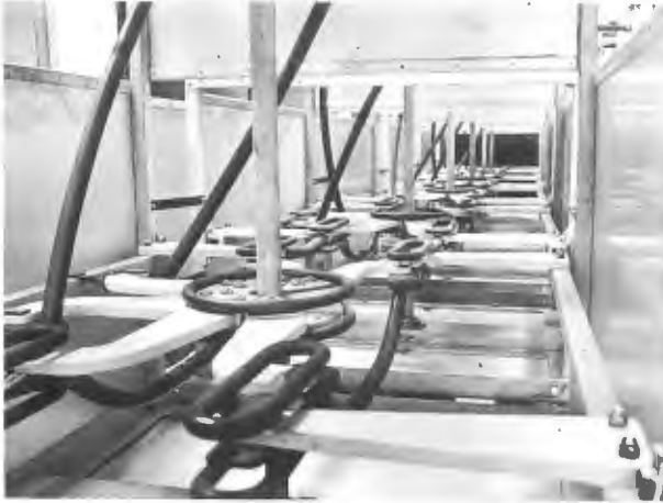
Figure 48.7 Transmission line switches
