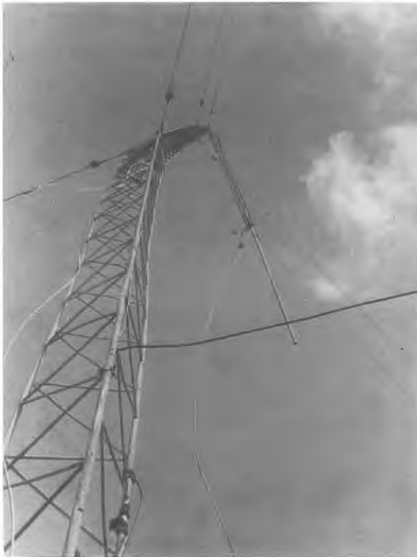
Figure 43.17 Damage to structure following failure of guy
