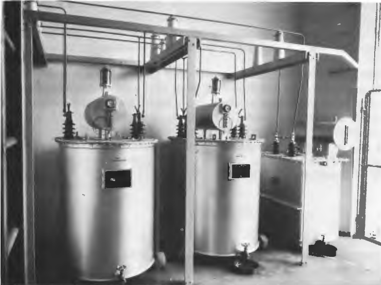
Figure 36.1 Typical oil filled vault equipment fitted with conservator tank and dehumidifier
