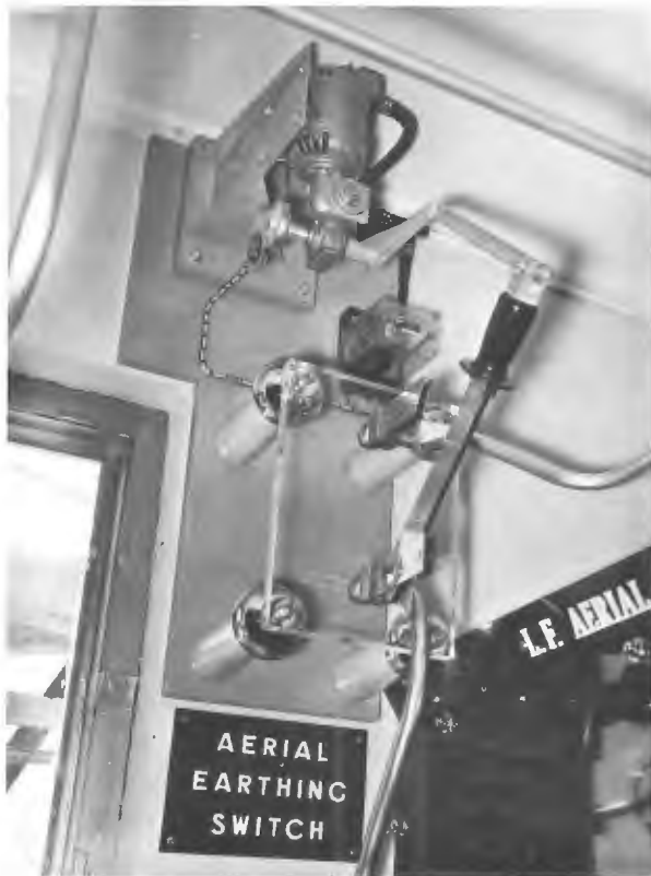
Figure 26.8 Remotely operated earthing switch
