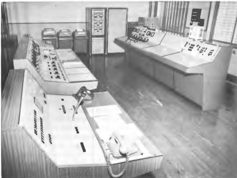
Figure 16.1 Control room of broadcast station equipped with digital control system
