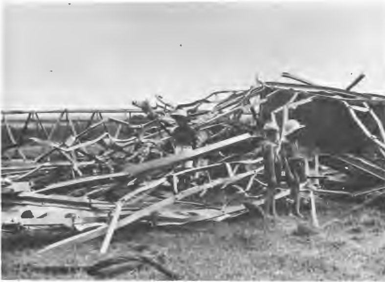
Figure 40.3 Damaged 160 m top loaded mast after collapse
