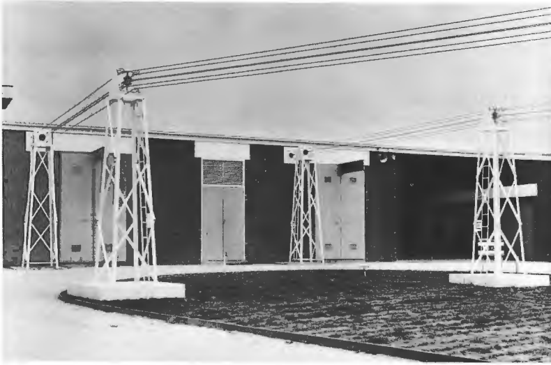
Figure 28.3 Transmission lines crossing site road
