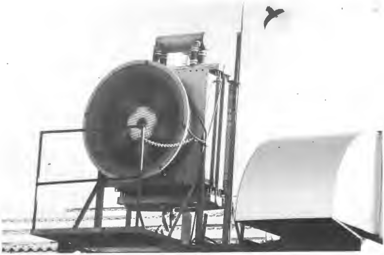
Figure 42.6 Roof mounted type steam condenser
