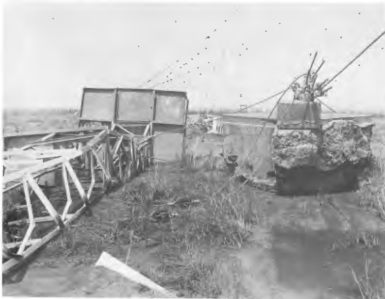
Figure 43.12 Guy foundation block pulled out of the ground
