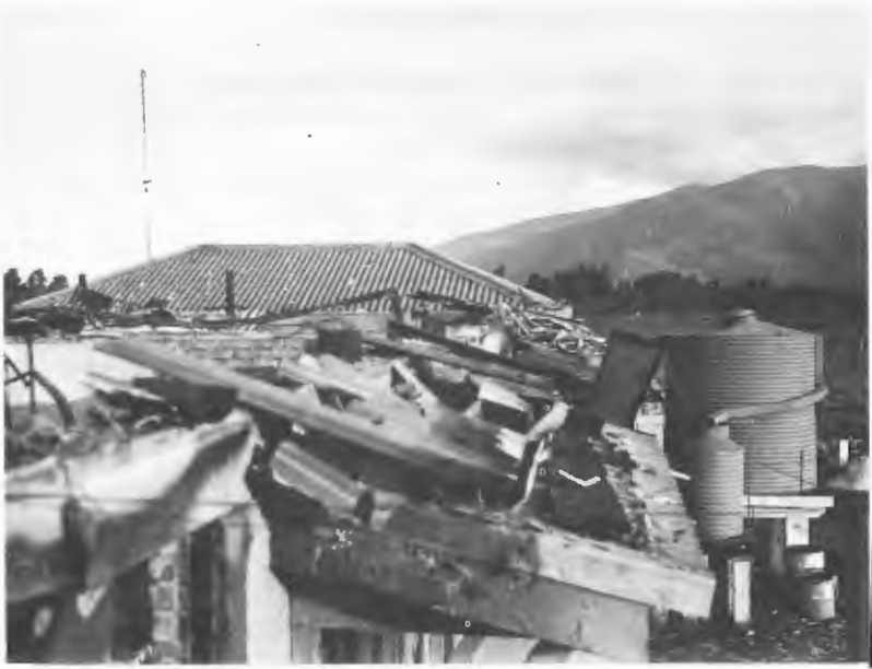
Figure 33.2 Damaged transmitting station building
