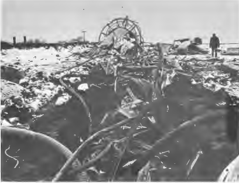
Figure 43.21 Damaged cables and waveguides (Courtesy Construction News)
