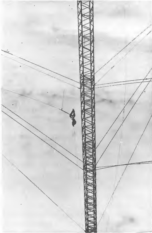
Figure 30.3 An unsafe practice during mast erection
