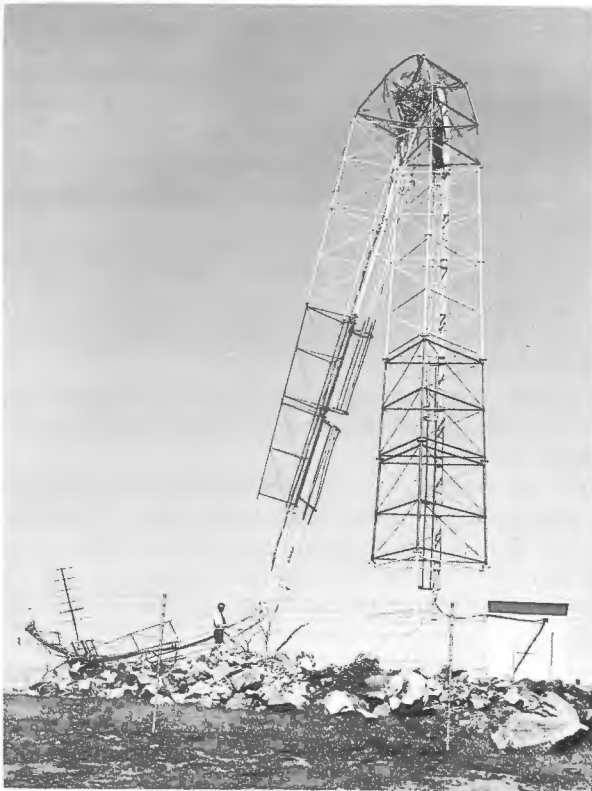
Figure 43.27 Damaged base station tower
