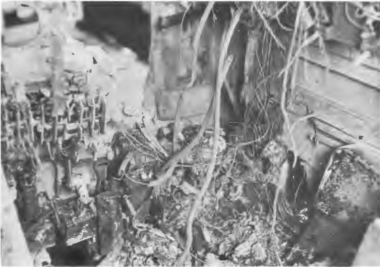
Figure 31.1 Polyvinyl chloride insulation burnt out in transmitter fire
