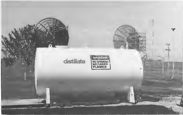
Figure 33.4 Temporary distillate storage tank
