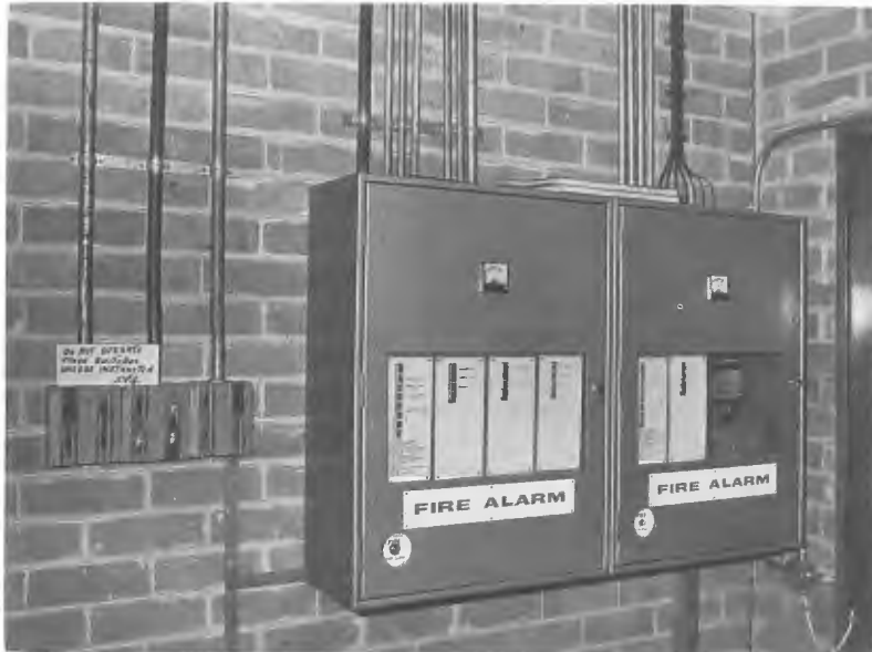
Figure 34.6 Typical fire alarm indicator panel
