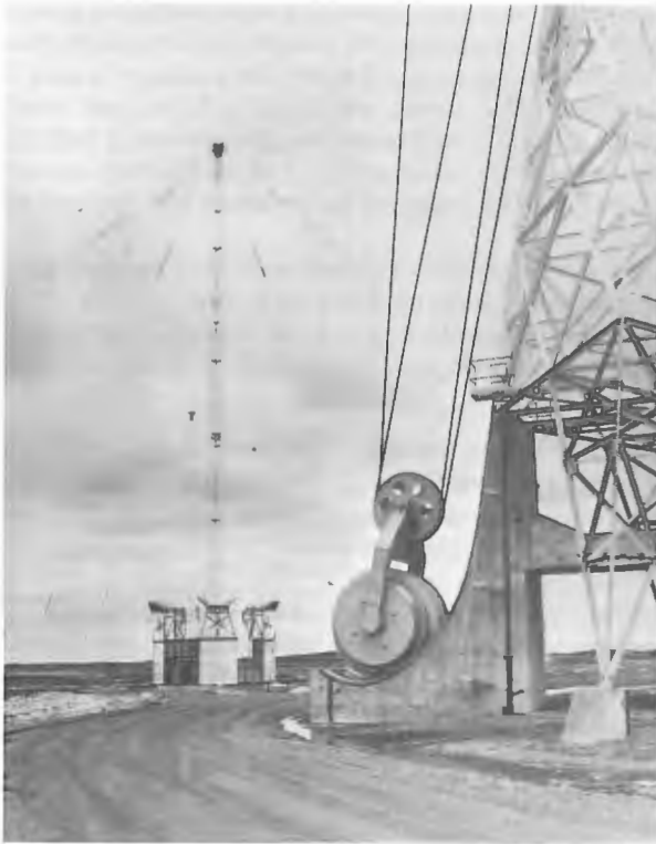
Figure 43.3 V.L.F. antenna counterweight system. (Courtesy US Navy)
