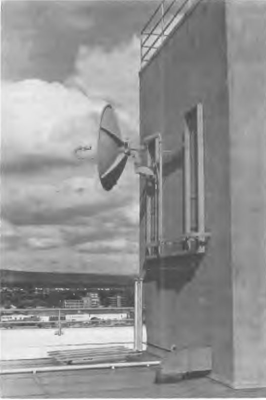
Figure 44.8 Antenna mounted on wall of building
