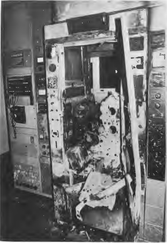
Figure 39.1 Front of damaged transmitter
