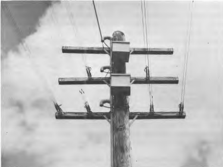
Figure 41.6 Balanced to unbalanced transformer boxes
