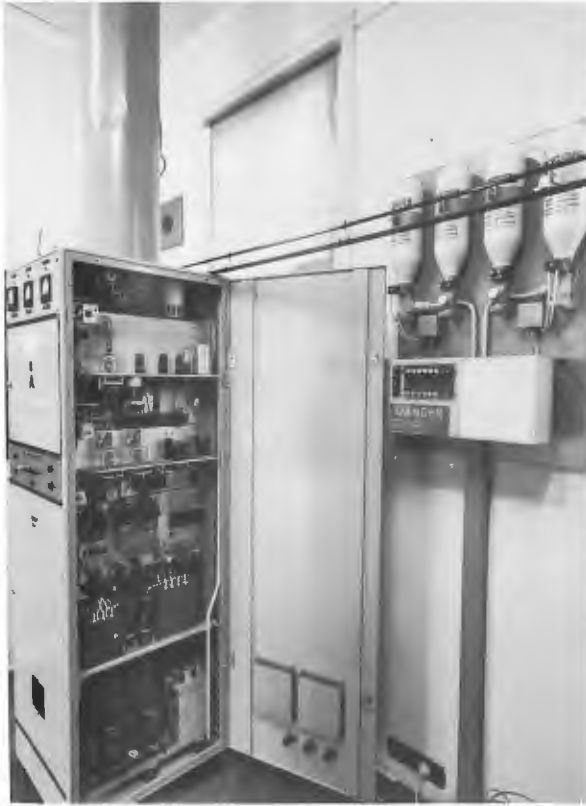
Figure 34.3 Automatic b.c.f. system fitted to a broadcast transmitter
