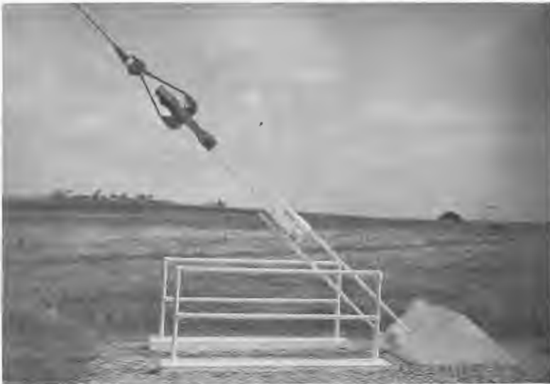
Figure 40.9 Guard rails for protection of guy
