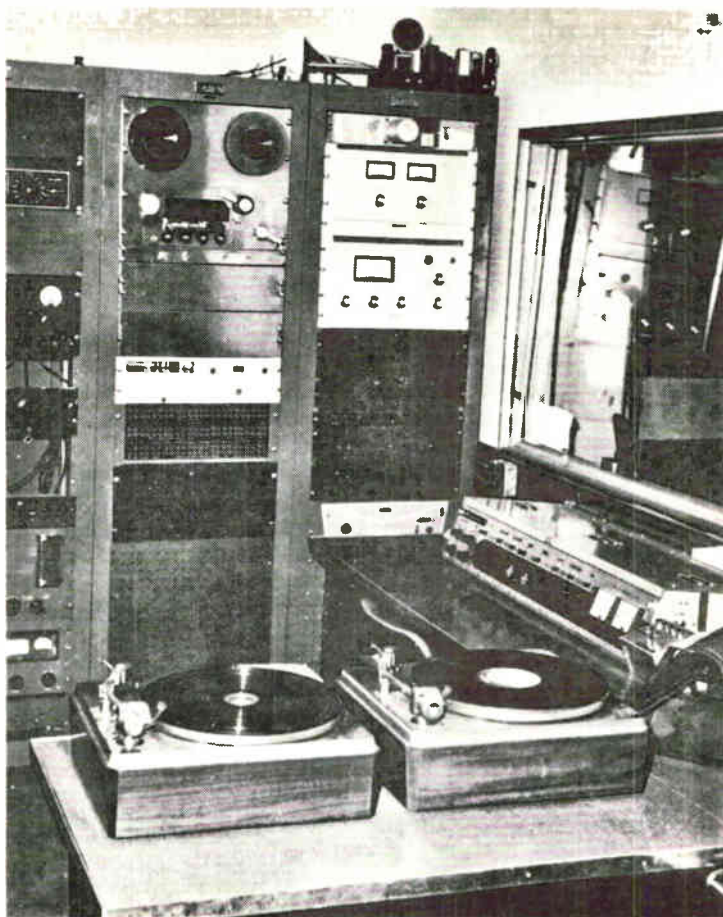
Fig. 1. View of transmitting studio, showing console, turntables, and rack equipment.
