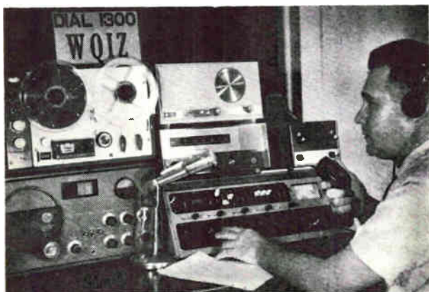
Author Jones in news room, which is separate from main control room and has facilities for taping of news and editing, or direct on-air feeds. Remote news transceiver is at upper right.
