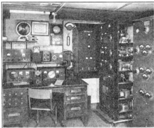
Figure 2. Amateur radiophone station W9NLP of Chicago, a typical high power installation using "commercial" type construction.
