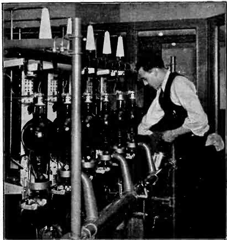
FIG. 10—View of 17,000 volt rectifier tube unit installation. (Courtesy Western Electric Co.)
